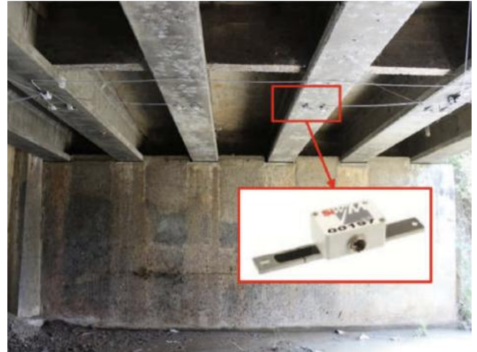
B-WIM instrumentation on the Pawiro Baru Bridge
