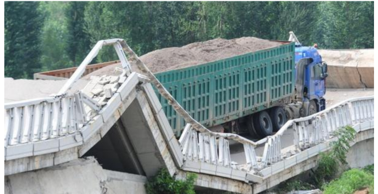
Bridge collapse due to overloading trucks (Deng et al., 2016)
