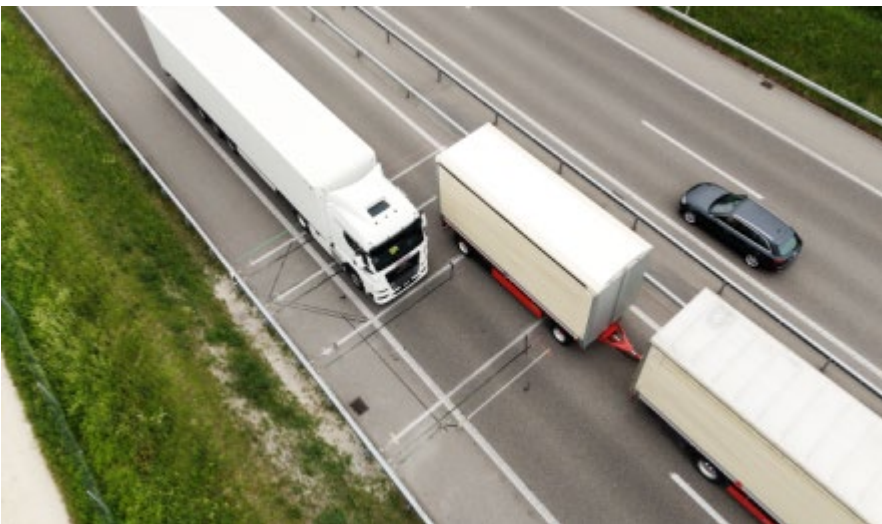
Kistler's KiTraffic WIM System installed on the A7 near Kefikon in Switzerland
