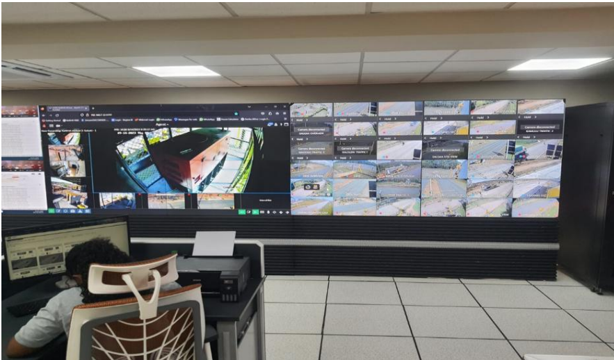
The Data Center at the KeNHA headquarters
