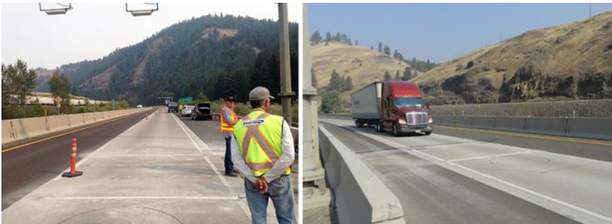
Intercomp strip sensors installed in Oregon, USA
