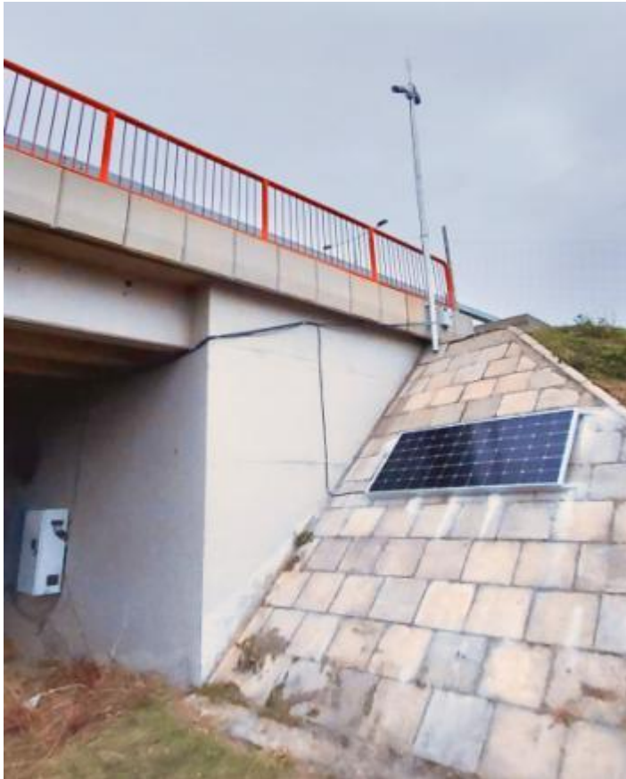
A solar panel powering a remote Cestel B-WIM system.
