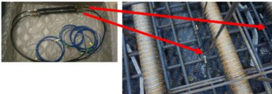
Optical fibre sensors attached to embedded reinforcement anchor.
