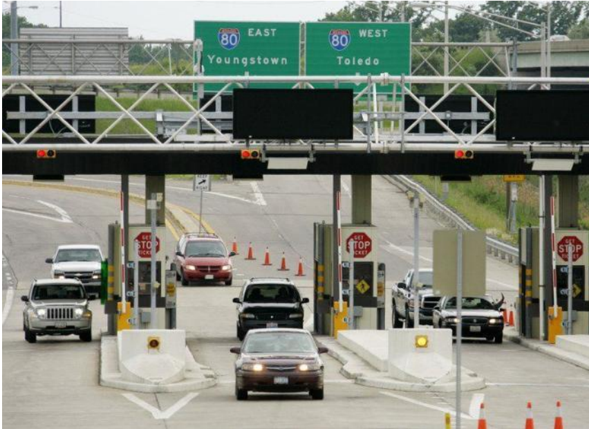
WIM systems at Ohio Turnpike toll station.
