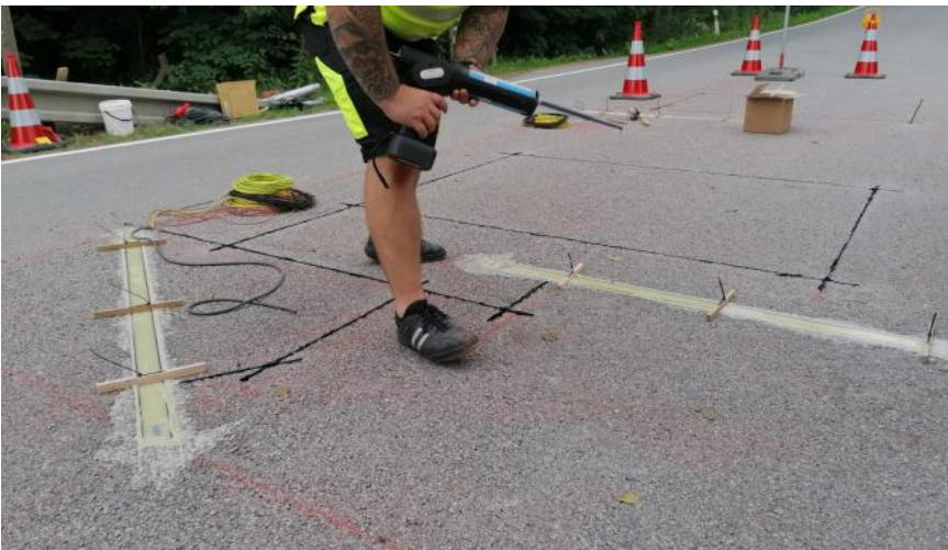
Installation of WIMTRONIC sensors.
