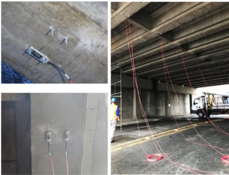
Strain gauge sensors installed under a bridge in Brazil
