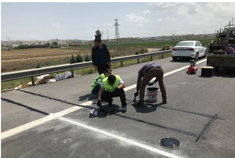
Installation of Lineas sensors in Turkey.
