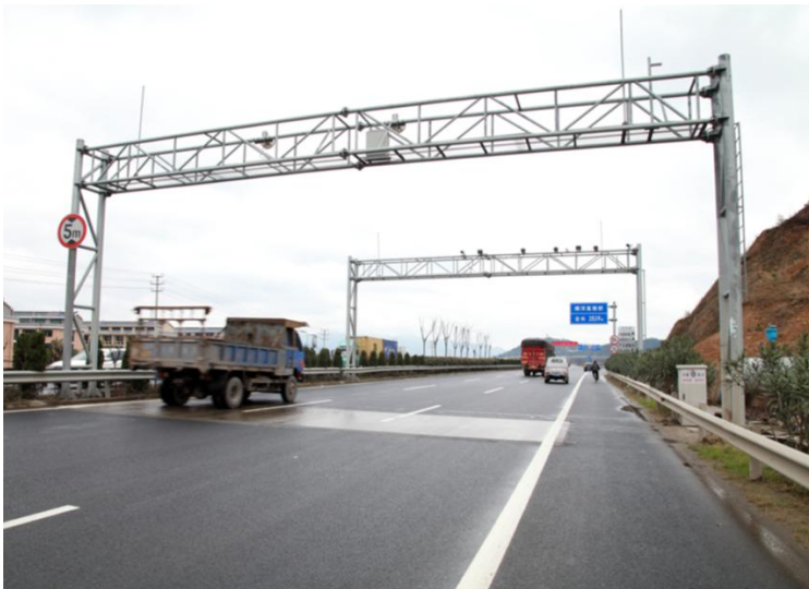
WIM Direct enforcement with LiDAR at Haining, China.
