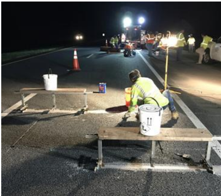
Installation of subsurface Quartz Sensors in Florida, USA
